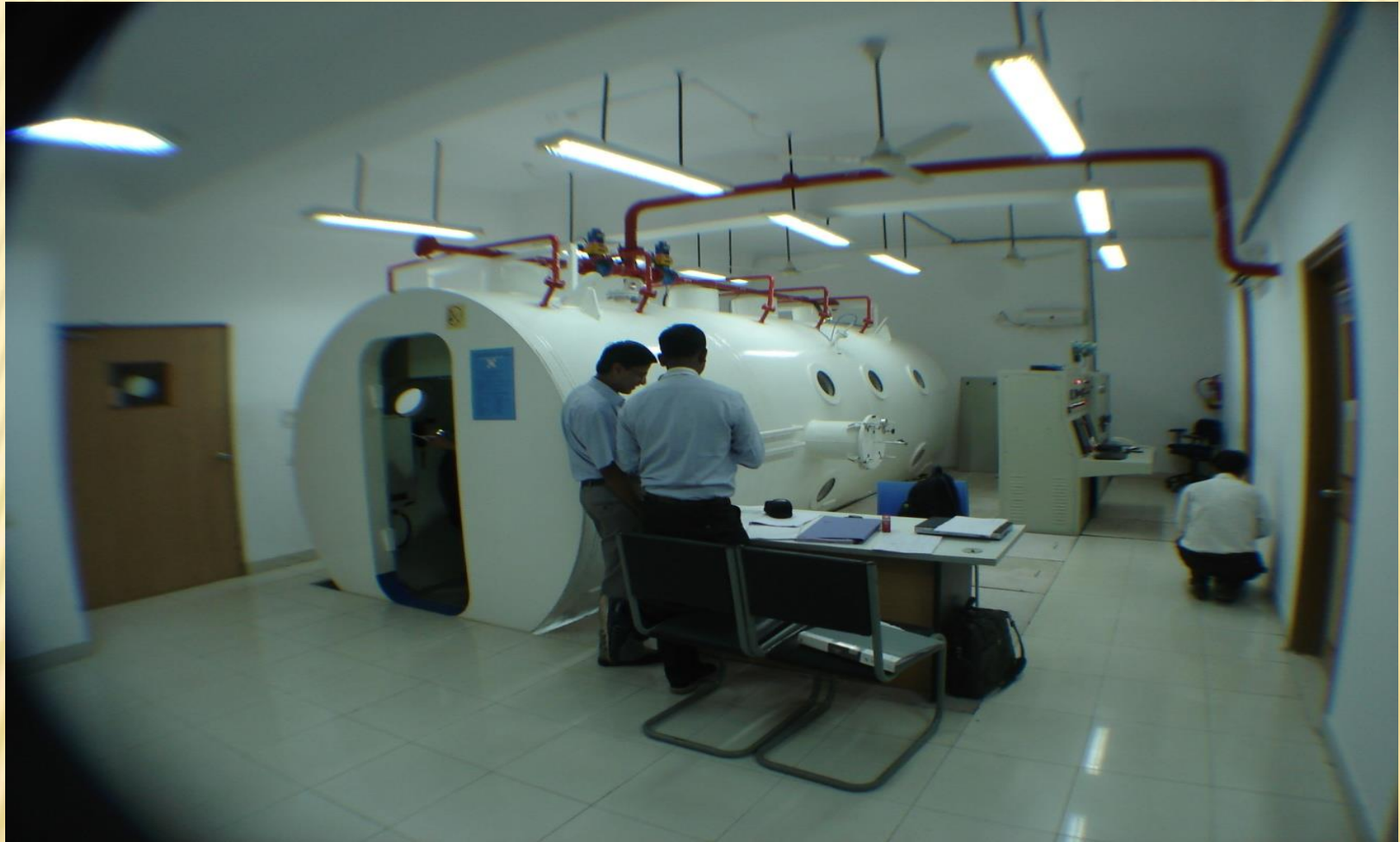
HBO CHAMBER AT GODREJ HOSPITAL , MUMBAI
